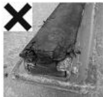
Damage to the End of the Rubber Strip.
