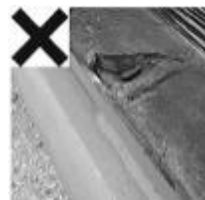
Damage along the length of the Rubber Strip
